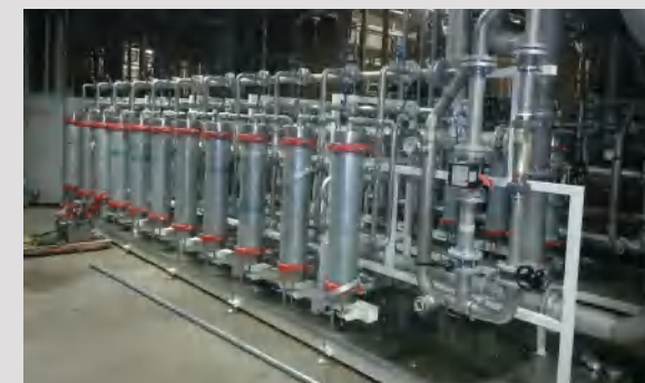
UF膜电泳漆浓缩
